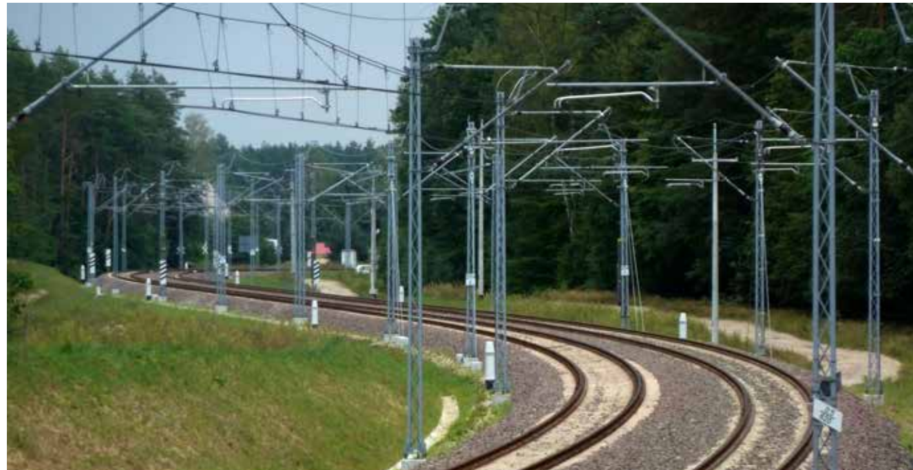
A railway line operated by the Polish state railway PKP PLK, featuring acoustic warning stations from the company NEEL to protect migrating animals from trains.
