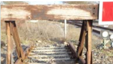
A track to nowhere: This is not what track connections should look like!
