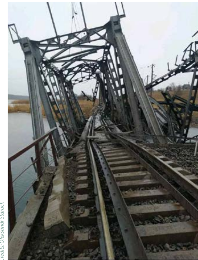
This photo of a railway bridge near Bacunivka / Vasylivka destroyed by Russians was published by the head of the Saporizhja district on March 1, 2022 on the Telegram channel.
